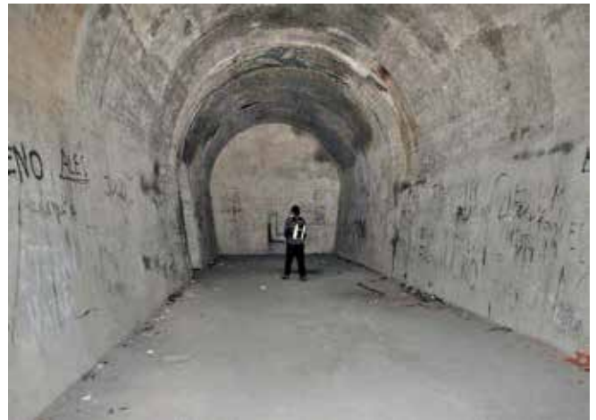
A large concrete lined chamber at the back of Bunker 2. The entrance on the left leads into the main tunnel network.
